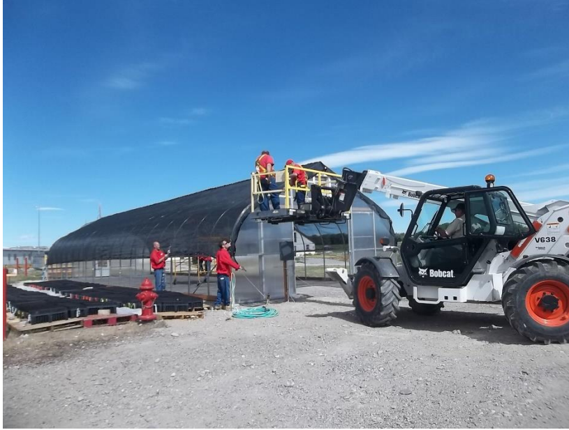
Figure 5 Sagebrush Canopy Cover: Wyoming Honor Farm inmates installing the shade canopy cover on the erected greenhouse structure. Photo by WY DOC 2019.
