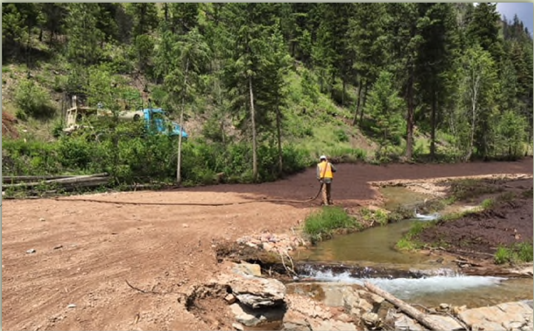
Flat Creek OU2 Project – Contaminated soils removed where possible and remaining contamination capped with imported soils
