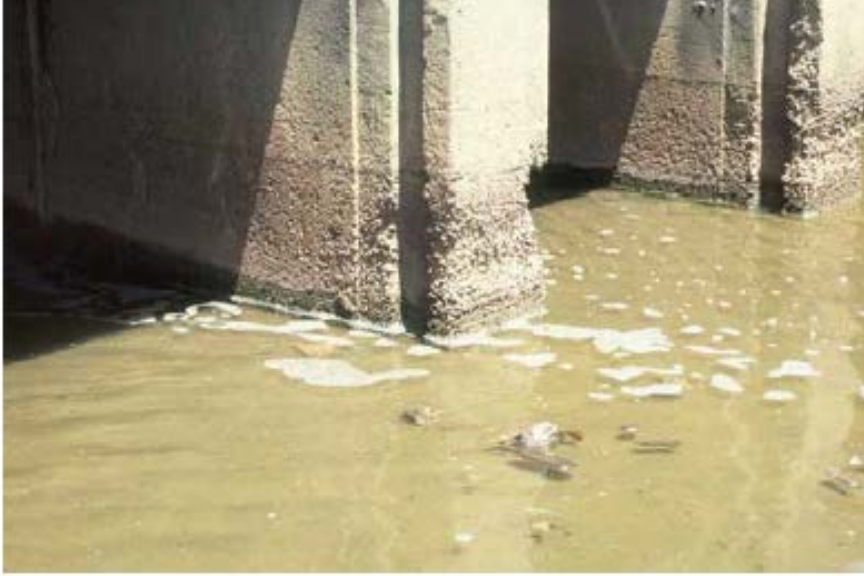
Figure 1: Concrete bridge pier damaged by acidic runoff from ASS.
