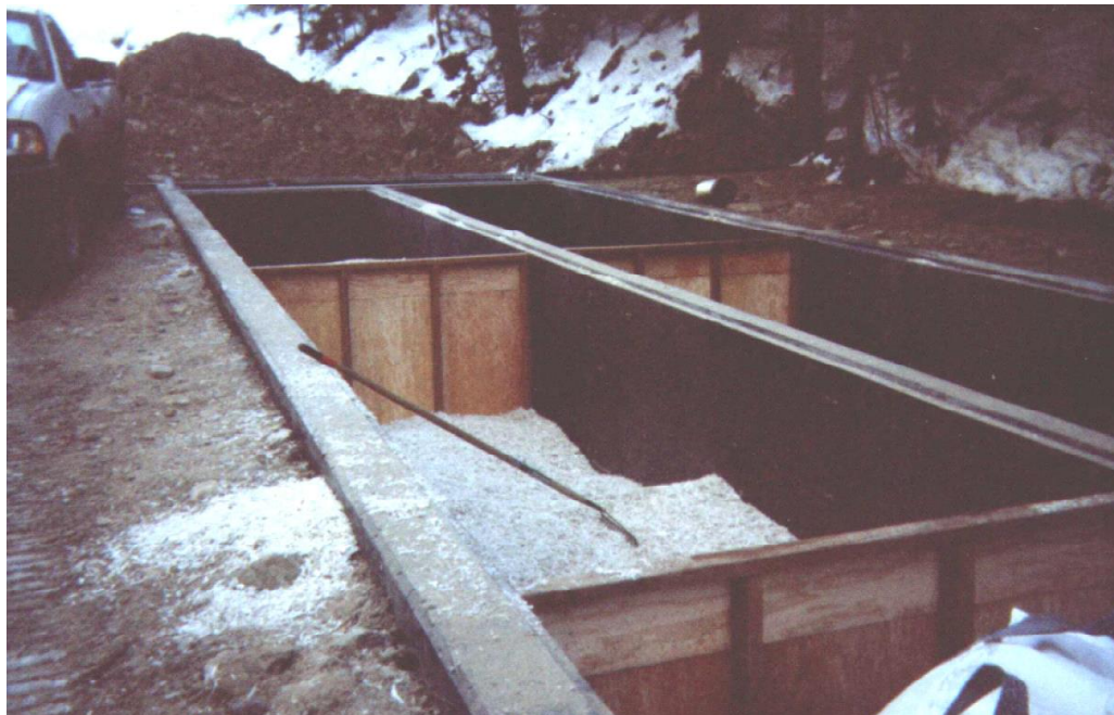
Figure 2. Installation of the Apatite II in the baffles of the PRB vault.
