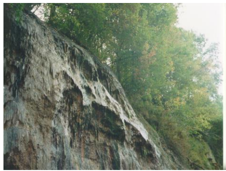
Figure 5b. Acid drainage seeping directly from the face of an abandoned highwall.
