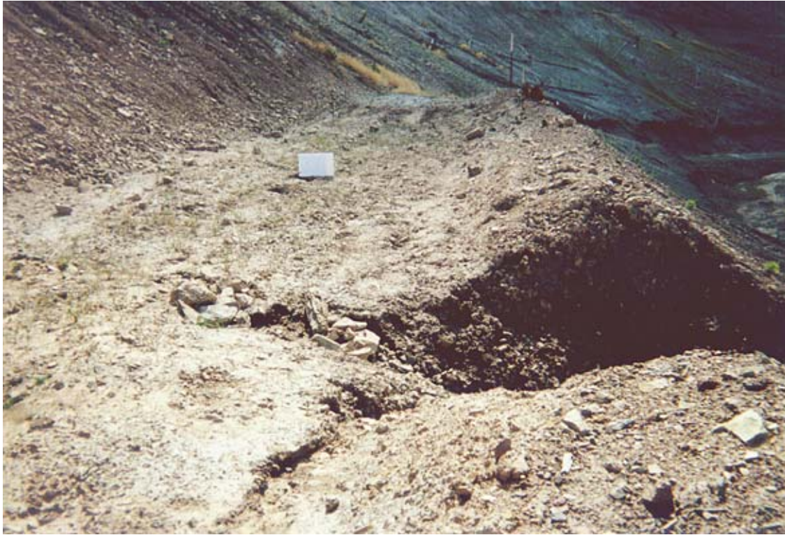
Figure 4. Terrace benches of the hillsides are relatively flat but cut and fill slopes are steeper than ambient slopes creating difficult revegetation conditions both above and below the benches. Most benches are intact. However, as shown here, water pools in places, saturating underlying soils and overloading the bench. This can produce mass movement and further gully down-cutting along the fill slope (photo taken in 1997).
