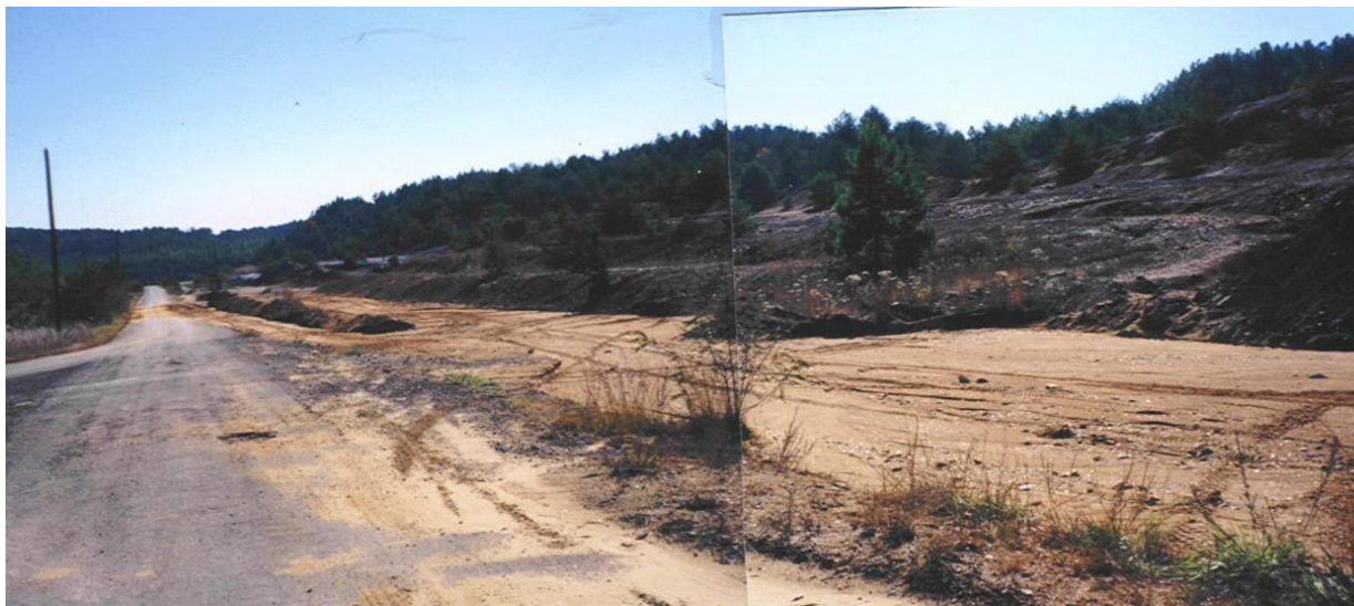
Figure 3. Silt from eroded areas at wetland construction site (well above flood plain).
