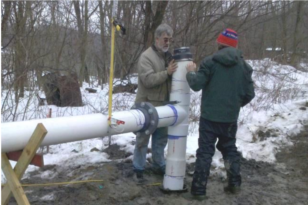
Figure 3. Flow rate measurement device (Test 2 installation shown) Orifice plate (in gray flange) and manometer (left of flange)
