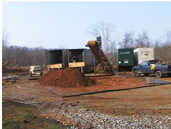
Figure 6. The two sludge storage tanks (right), two frame filter presses (left), conveyor, and product.
