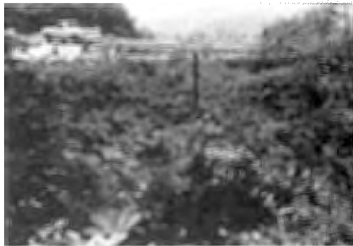
Figure 3. The sequence of three photographs below show the before, during, and after of a haul road stream crossing excavation.
