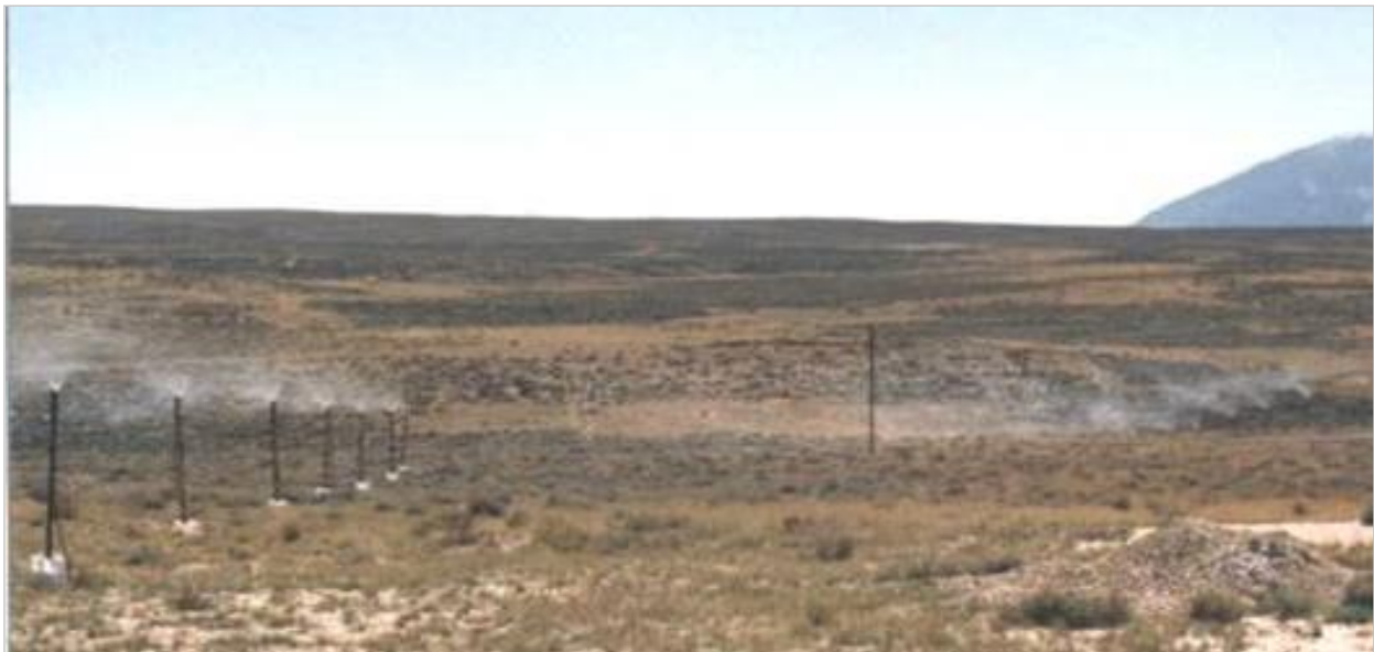
Figure 11. Spray System for Dispersal and Evaporation of Ground Water after Treatment, September 23, 1988.
