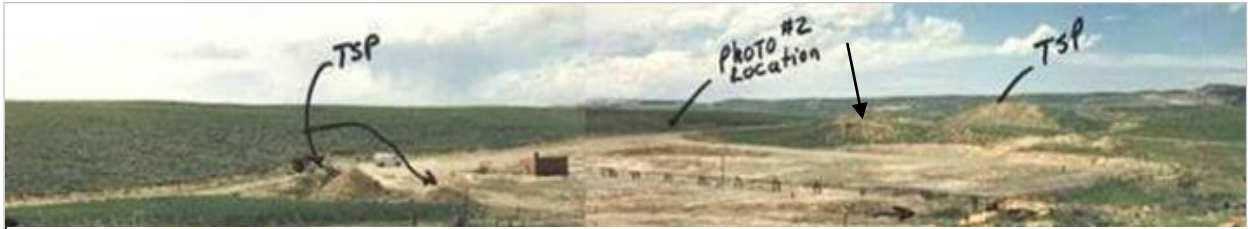
Figure 4a. Facilities Area at the RD15 Site after removal of buildings and most equipment, June 18, 1991, looking northwest. TSP refers to Topsoil Stockpile. The "Photo #2 location" is a reference to another photo, not included in this paper, taken during the June 1991 inspection.
