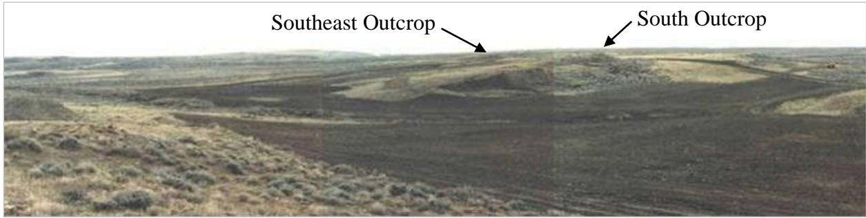
Figure 5a. RD15 Site after completion of grading and application of most of the topsoil, October 12, 1993, looking southeast.
