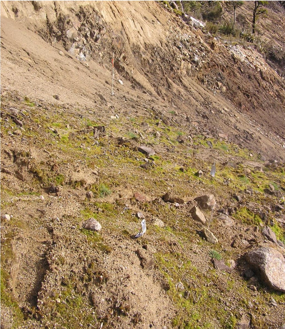
Figure 4. Erosion runnel on the granite veneer site with adjacent moss growing in the protection provided by a large boulder.
