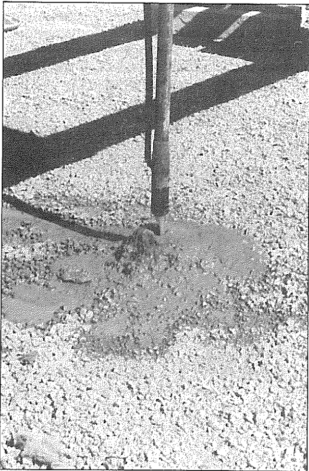
Figure 2. Nozzle used for application of sodium silicate and cementitious grout in column construction.
