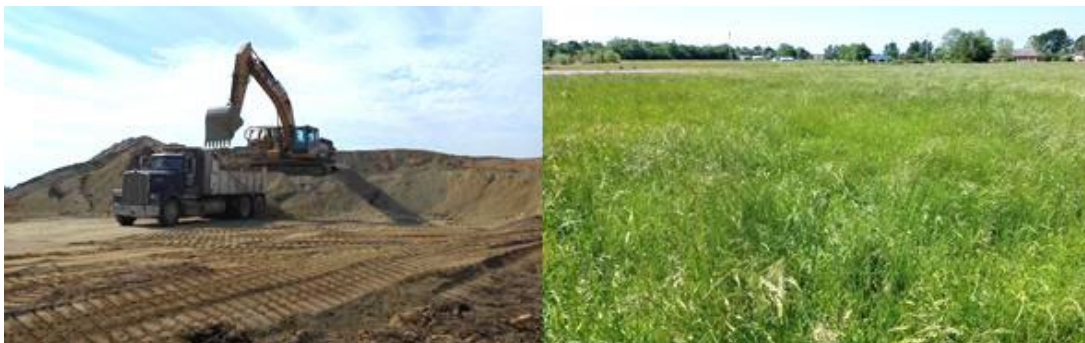
Figure 4 This site was included as a post-remediation site in the bird study – great before and after example of reclamation.
