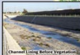
Channel Lining Before Vegetation
