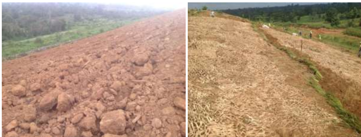
Figure 3. Scarification after TSP re-instatement (left), BGTs installation and vegetative planting of Vetiver grass stalks (right).
