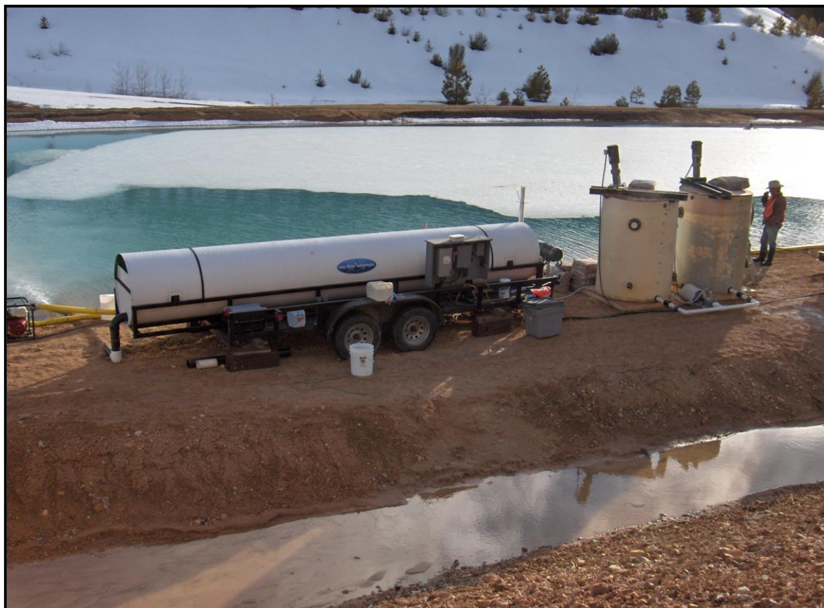
Figure3. RCTS system at the Leviathan Mine.
